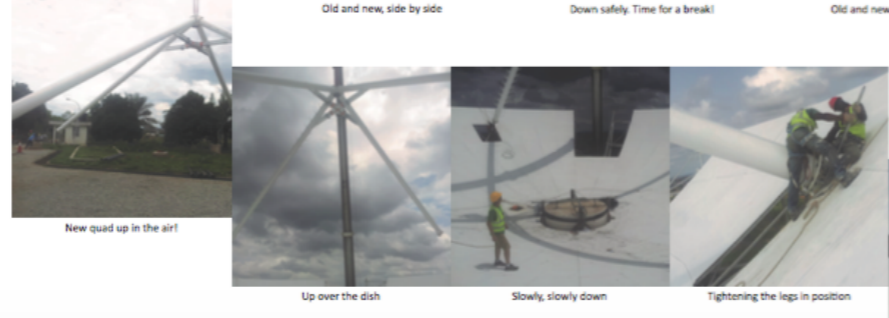
Old and new, side by side Down safely. Time for a break! Old and new Up and away! Getting ready to lift Bracing the old structure at its weakest points
