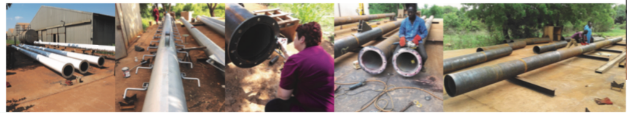
Done! Rungs, cross-brace attachments, and primer Visual inspection of flange welds Attaching end flanges Full lengths appearing!
