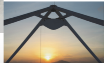
New quad up in the air! Up over the dish Slowly, slowly down Tightening the legs in position
