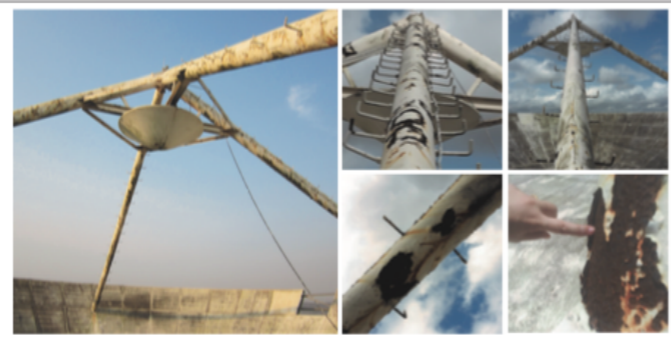
Original quadrupod structure. The quadrupod legs have to be rigid enough to ensure that the 300kg subreflector is held in the correct position, at the correct angle, in order to focus signals along the right path down the beam waveguide.
